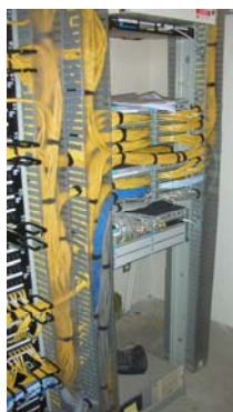
Data Closet After
