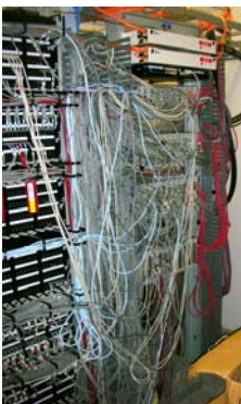
Data Closet Before
